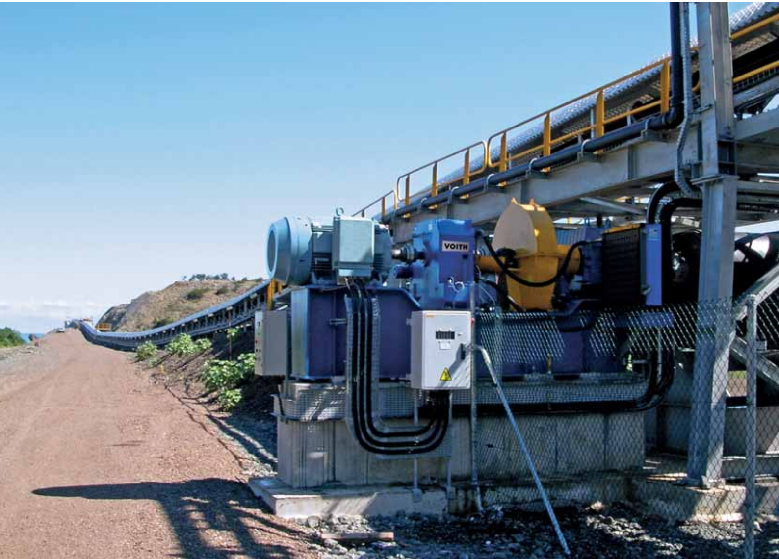
Fill-controlled coupling in a belt conveyor drive
