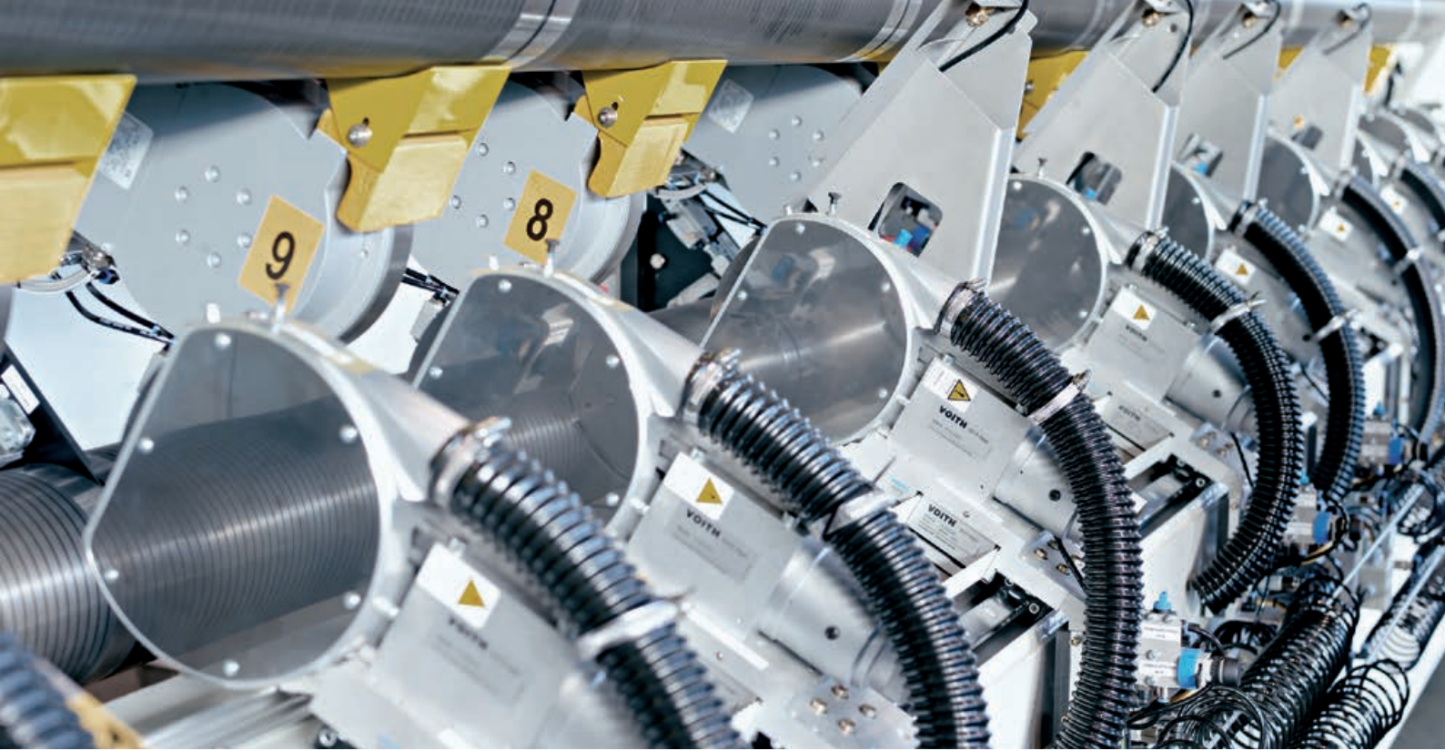
Slitter dust extraction system
